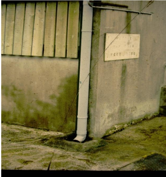
Gully with concrete surround to maintain clean and dirty water separation.
