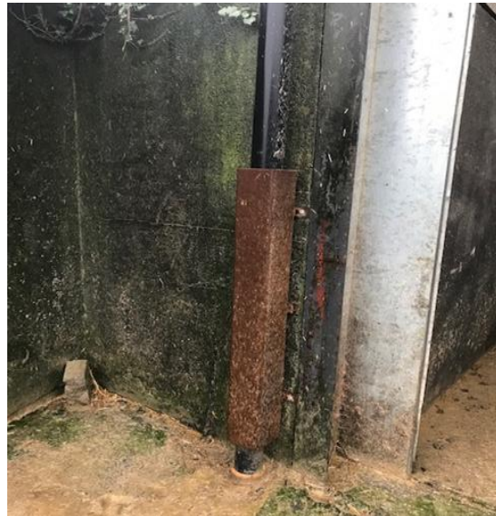
Downpipe direct to drain to avoid contamination. Note damage protection
